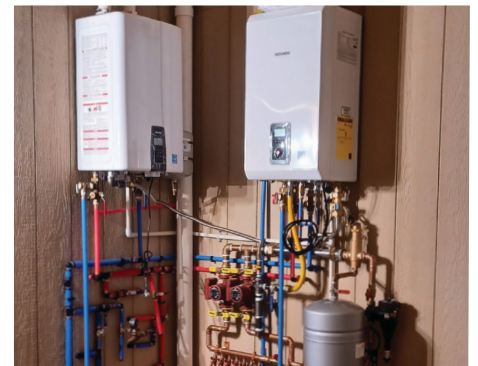
Triple H Plumbing offers Navien Tankless Water Heaters, providing endless hot water & energy savings up to 40%
